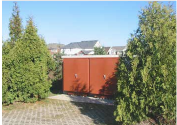
Image example of a Bell CUE unit partially screened within an easement adjacent to a SWMP facility.
